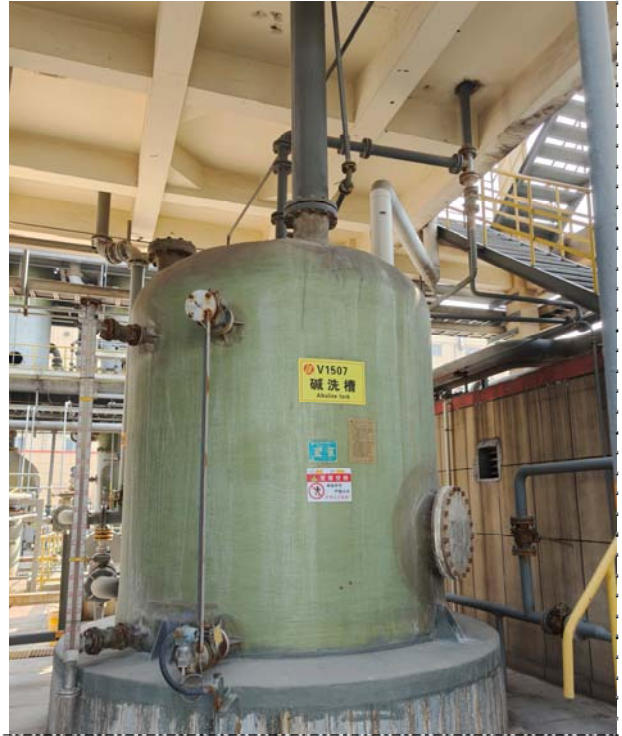
焚烧炉废气碱洗槽
