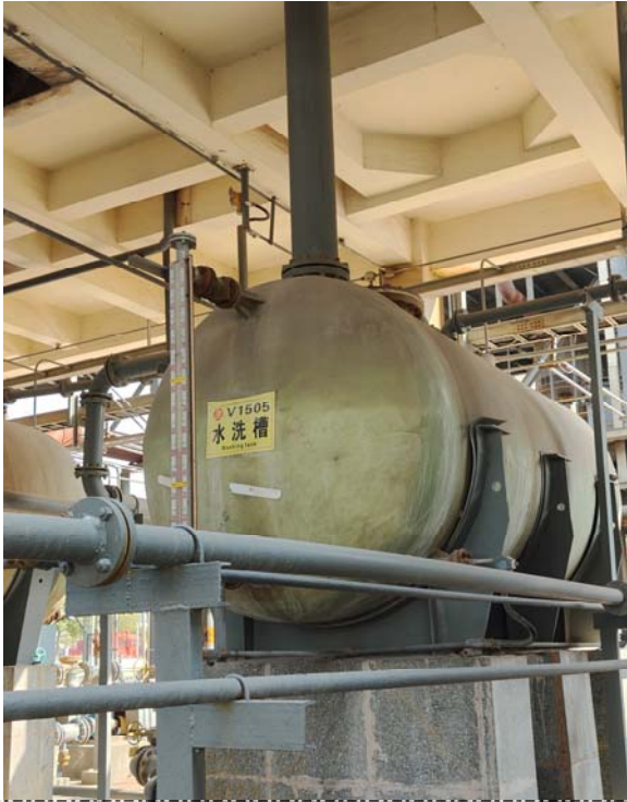
焚烧炉废气水洗槽
