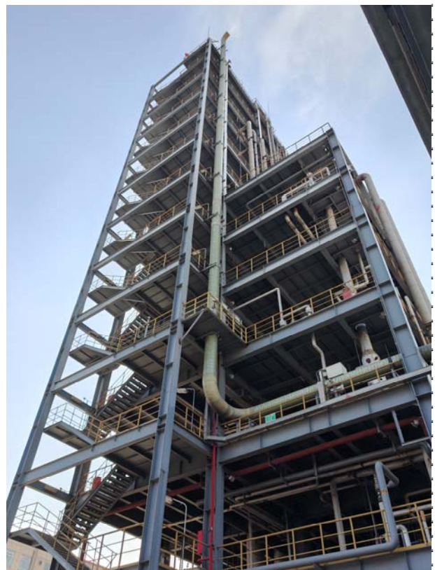
焚烧炉废气排气筒
